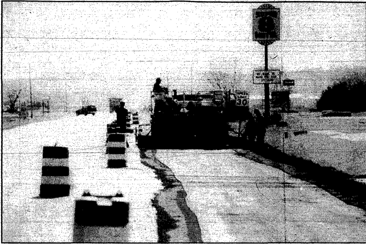
Dobson Brothers Construction Company worked on a temporary road east of town on Highway 35 in conjunction with the road construction that occurred in Wayne this summer.
